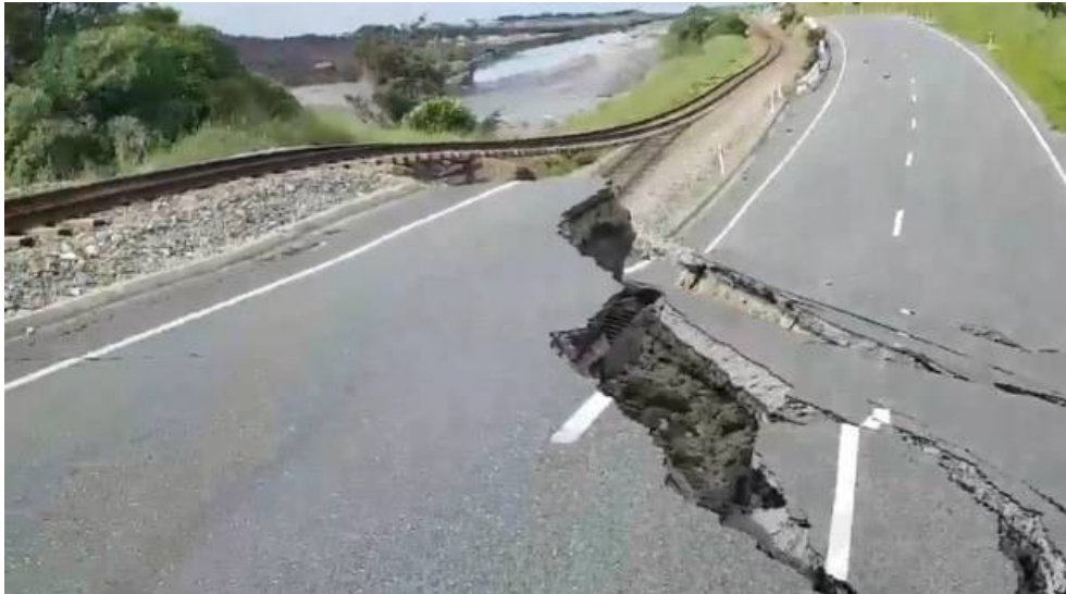
Figure 2: SH1 and the Rail Line Near Kaikoura (Source: Twitter, 2016)
