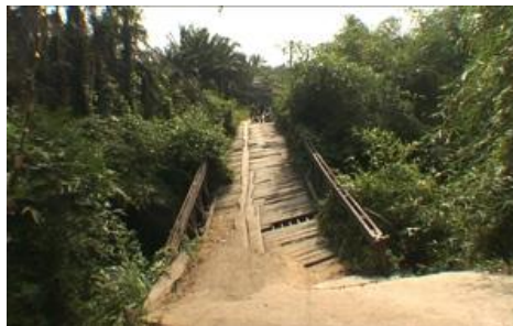
Diagram 4. Collapsed bridge, Akwa Ibom district, Nigeria
